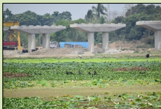
Figure 4: Construction work poses a growing threat to the wetland ecosystem. This picture was taken at Mathura Beel near Kanchrapara.
